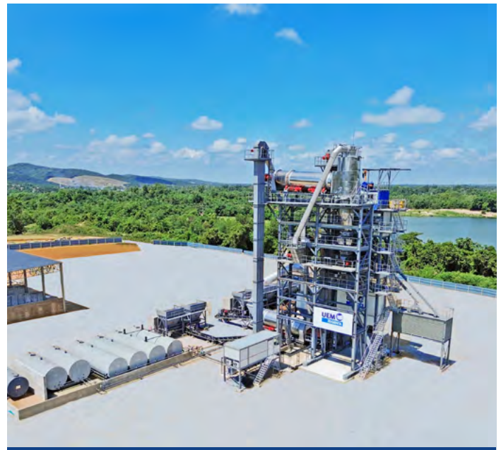
Asphalt Premix Plant with Recycling Facility in Tapah
